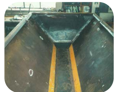
Aggregate sieve abrasive blast cleaned and relined with 3 coats of 209 EIP PU
