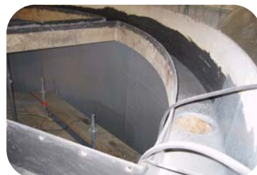
Chemical powder process vessel and chute were lined with 3mm of 209 EIP PU.
